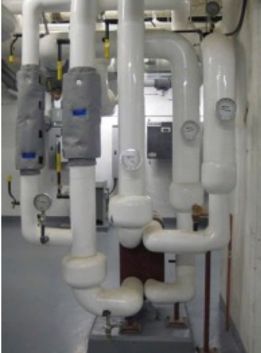
Typical Energy Transfer Station – Courtesy of FVB Energy
