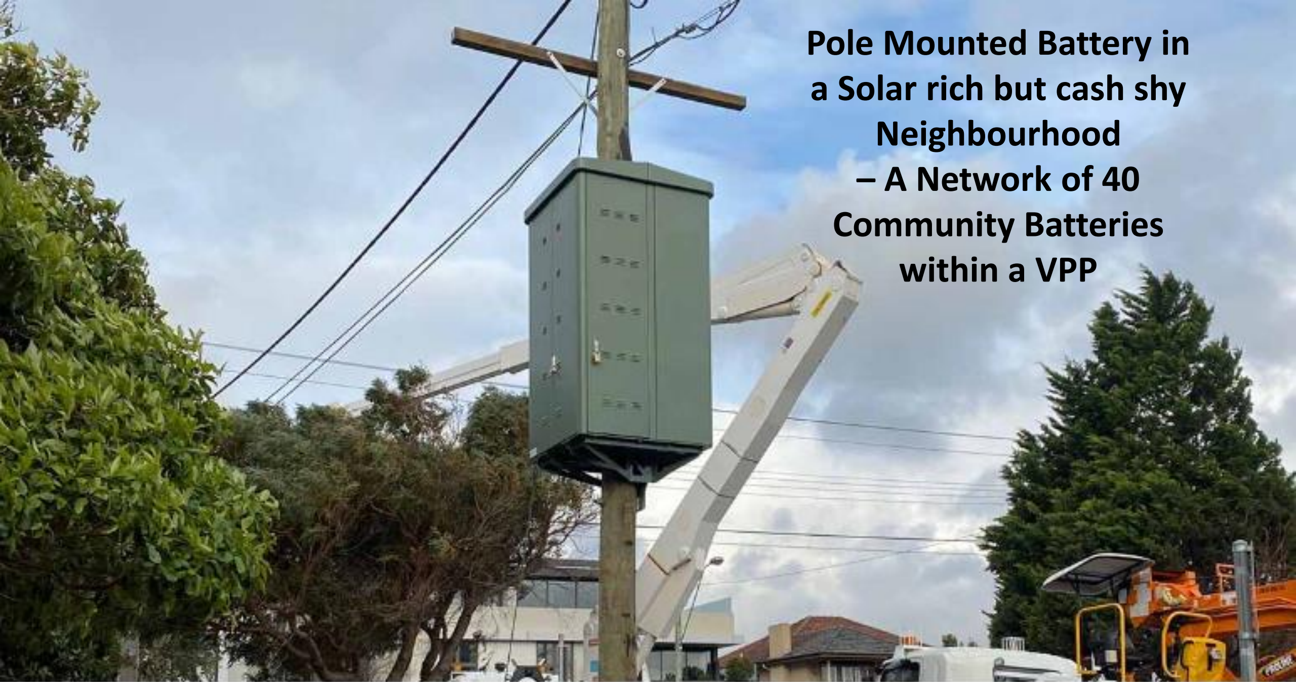
One of 40 community batteries to be distributed as part of a United Energy trial in Victoria.
