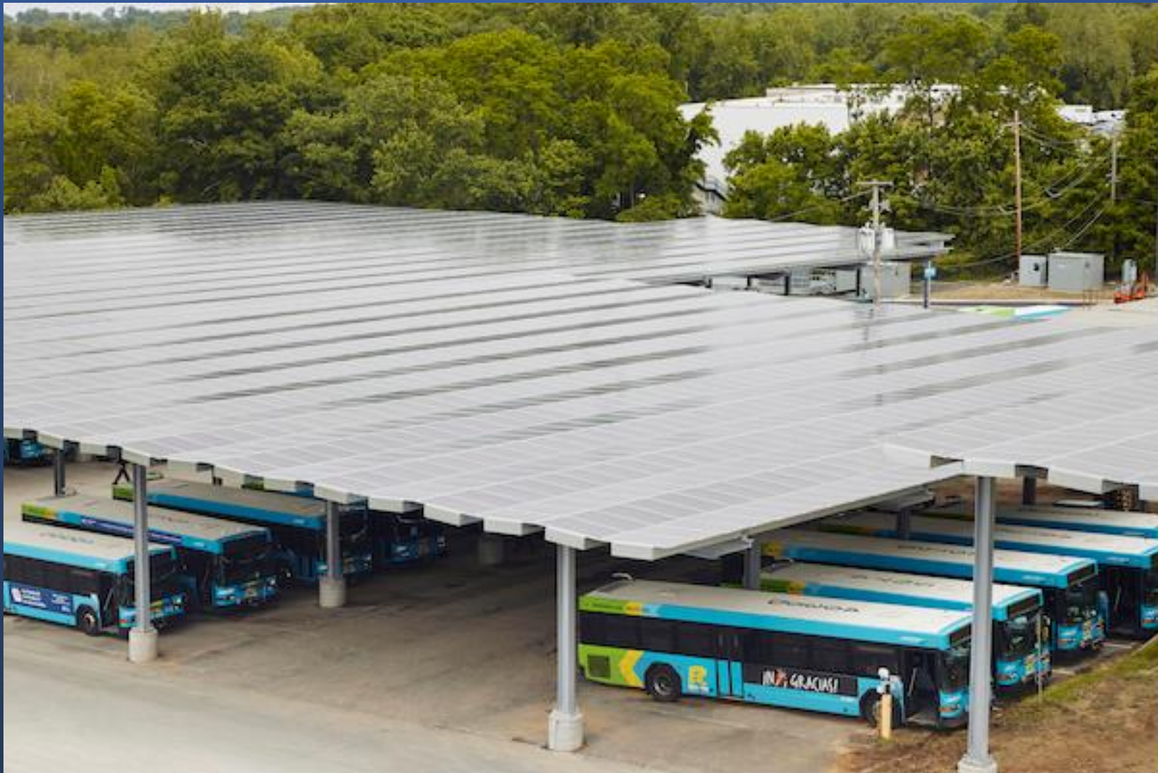
Solar canopy at Brookville Bus Depot in Montgomery County. The microgrid for the Depot includes a 1.6 MW solar PV array and a 3 MW Battery Energy Storage system. Image courtesy of Schneider Electric.
