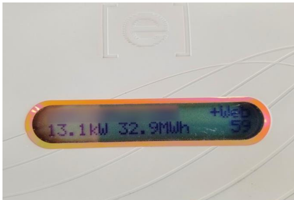
Figure 3: Enphase Microinverter Monitor Display
