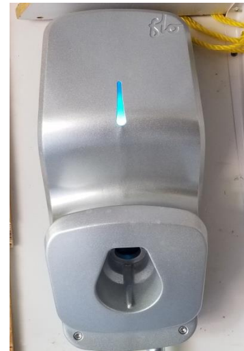
Figure 6: EV Charging Station
