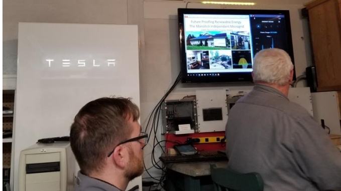
Figure 5: Tesla Powerwalls in the Control Room
