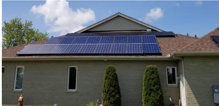
Figure 2: A Section of Dr. Hunter's Solar Panel Array
