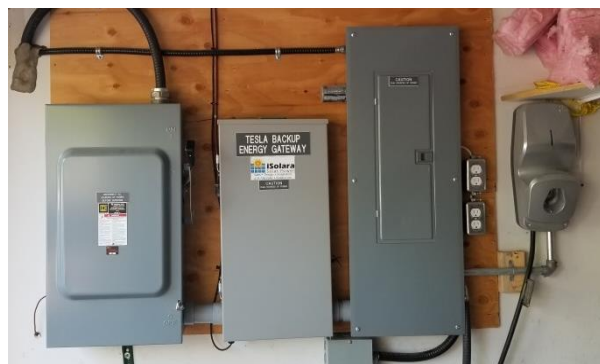
Figure 4: Switch, Gateway, and Breaker Boxes
