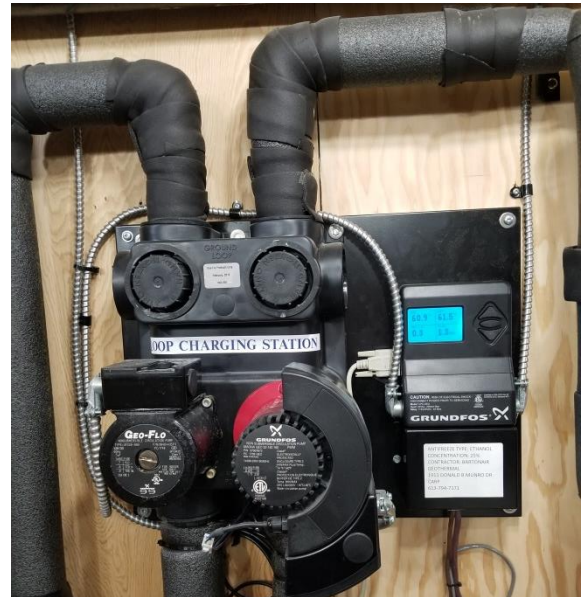
Figure 9: Loopanol Pumps and Meter
